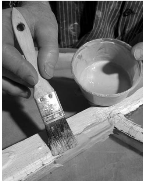
Figure 5 Liquid putty is brushed into small cracks in the front putty. This is a simple measure to delay ageing.
