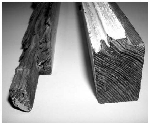
Figure 4 Window sections 15 years old (left) and 150 years old (right).
